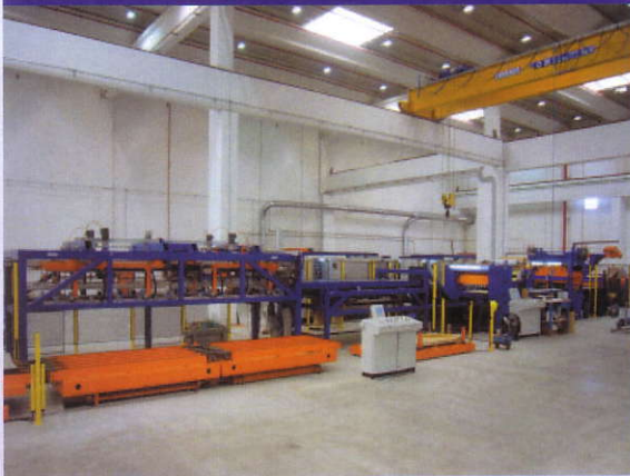
LEVELLING AND CUT-TO-LENGTH LINES
